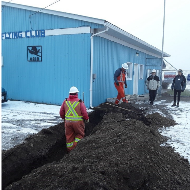
Fortis Installing Gas Line. Alison Crerar and Edit Schleiss cheer them on.
