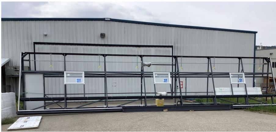
Wyatt McMurrery has bought and is renovating the big hangar off Taxiway Charlie. The new door is waiting to be installed.
